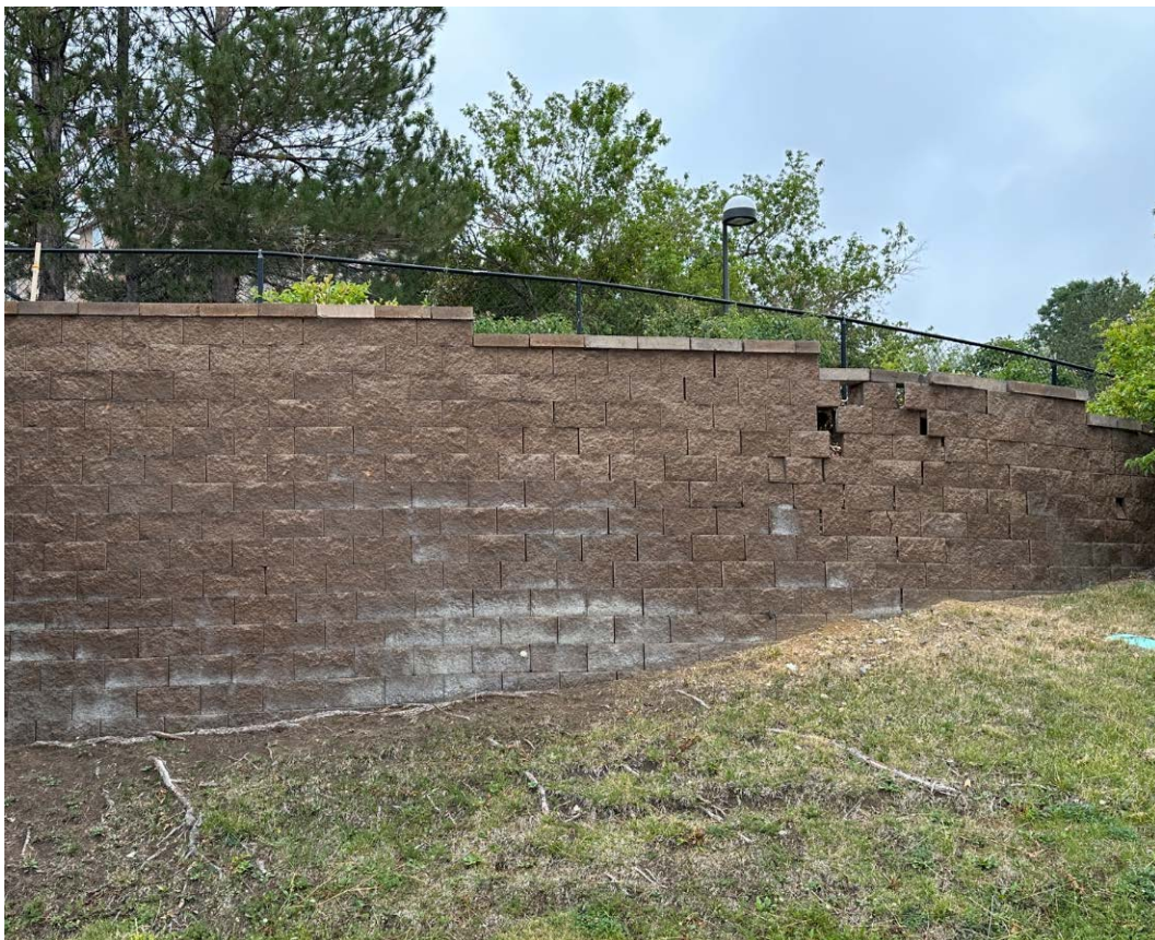
Figure 1 - Current Wall Condition
